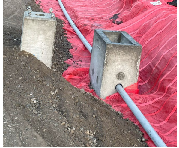
Lamp post foundation and conduit
