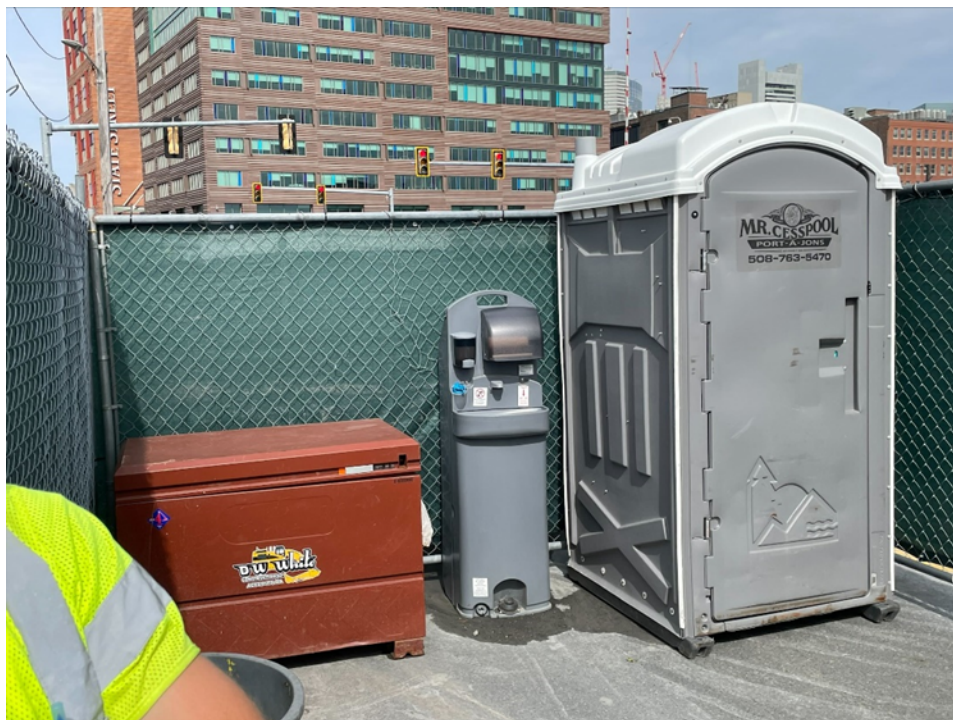
Personnel decontamination station in TSCA Area
