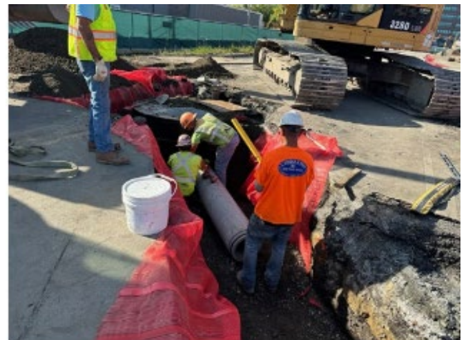
Drainage in roadway in TSCA area over marking layer
