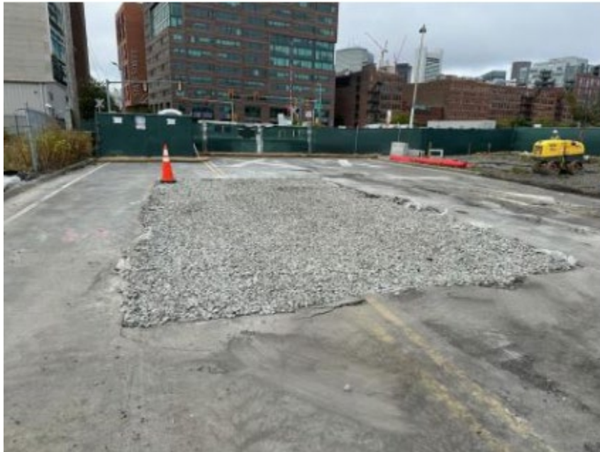
Expanded Truck Decontamination Wash Pit
